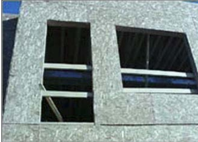
Figure 35 - Guardrails protecting window openings.
