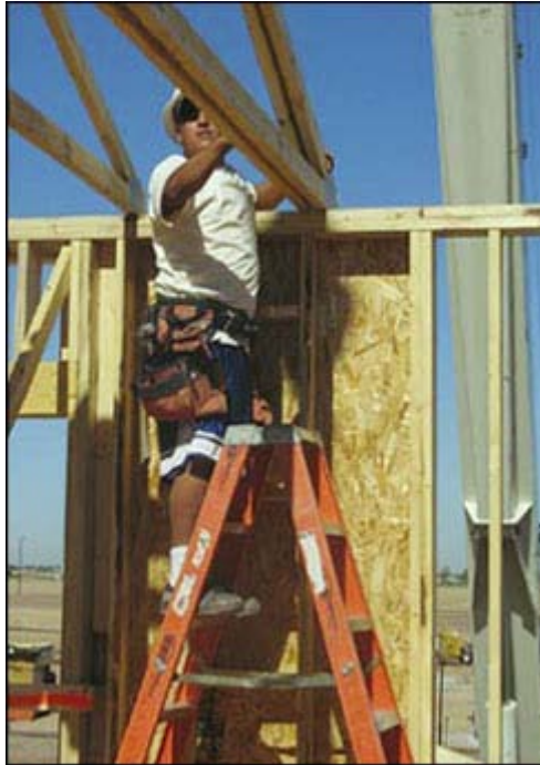
Figure 3 - Platform ladders can be set up inside a structure and used to install roof trusses.
