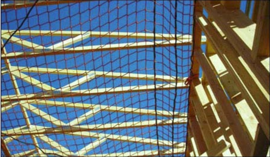
Figure 7 - An example of a safety net system.
