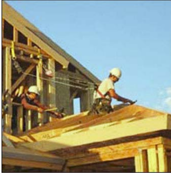
Figure 5 - Strap anchors providing anchorage for three personal fall arrest systems.
